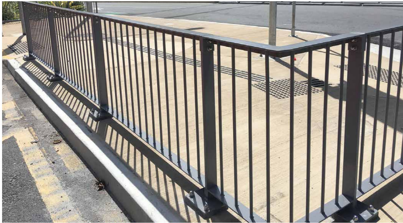
GOLD COAST LIGHT RAIL - ROAD SAFETY BARRIER FENCING; INSTALLED FOR BMD AS PART OF THEIR DELIVERY OF THE LIGHT RAIL INFRASTRUCTURE.
